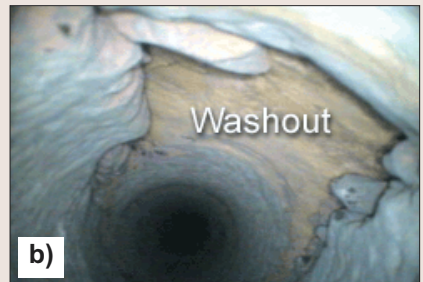
Figure 5. Images of unconsolidated rock layers from boreholes. Washout condition is evident in (b).
